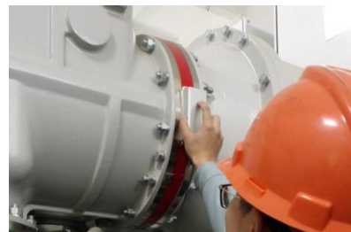
GIS field partial discharge test
